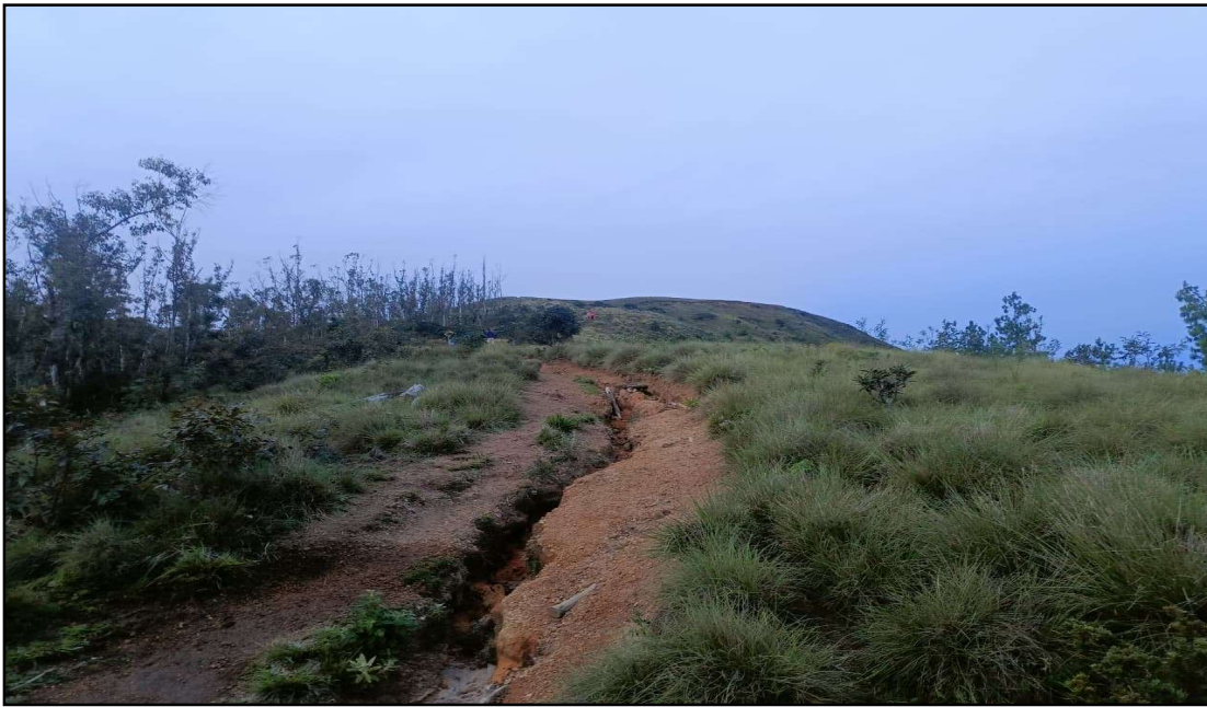
Plate 2. Eroded section of the Meeshapulimala trekking trail shows unstable walking conditions
